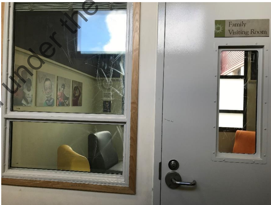
Photo: Family visit room with graffiti on windows and door
